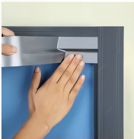
Window Frame Gap
