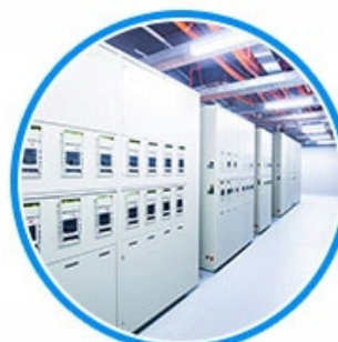
Industrial equipment testing
